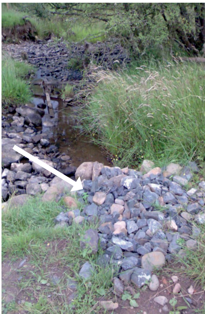
Figure 6: Completed abstraction point. Arrow indicates abstraction point inlet. Transfer pipe used at this site was 100mm diameter; this will vary from site to site.
