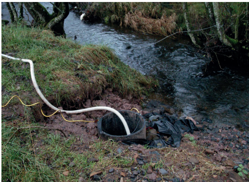
Figure 3: Abstraction point under construction to support a submersible pump with low level float switch. Abstraction sump chamber formed from pipe with diameter 450mm.
