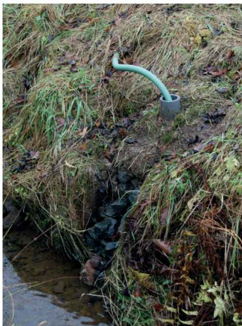
Figure 2: Abstraction point supplying a pasture pump. Pump inlet hose going into abstraction chamber fitted with a removable inlet screen. Abstraction sump chamber formed from pipe with diameter 150mm.
