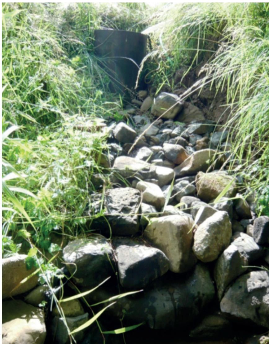
Figure 4: View from the watercourse of the completed abstraction point seen in Figure 3.
